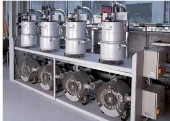
Central vacuum station
