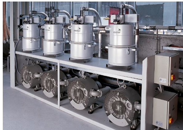
Central vacuum station
